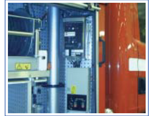
Mounted in fire truck
